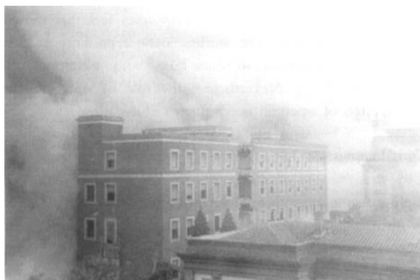
Figure 1 Cloud of dust produced the day of the controlled demolition of our maternity hospital.
