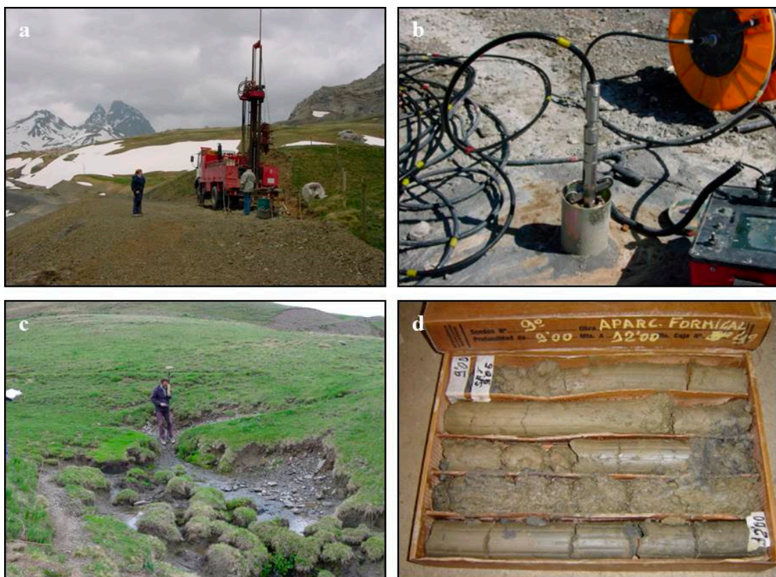
Figure 4. New geotechnical investigation works: (a) Borehole performance; (b) Inclinometer installation; (c) Inventory of water points; (d) Example of the Quaternary material obtained in the boreholes.
