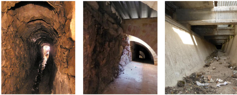
Fig. 3. Perimeter cavity on the outside face of the foundations: a) Church of convent of Santa Cruz la Real in Segovia, drainage, 2015-01-29; b) Parish church of Vall de Almonacid (Castellón), air cavity and rainwater harvesting, 2015-10-23; c) Church of San Salvador in Toro (Zamora), rainwater channel parallel to the air cavity, 2016-03-15.
