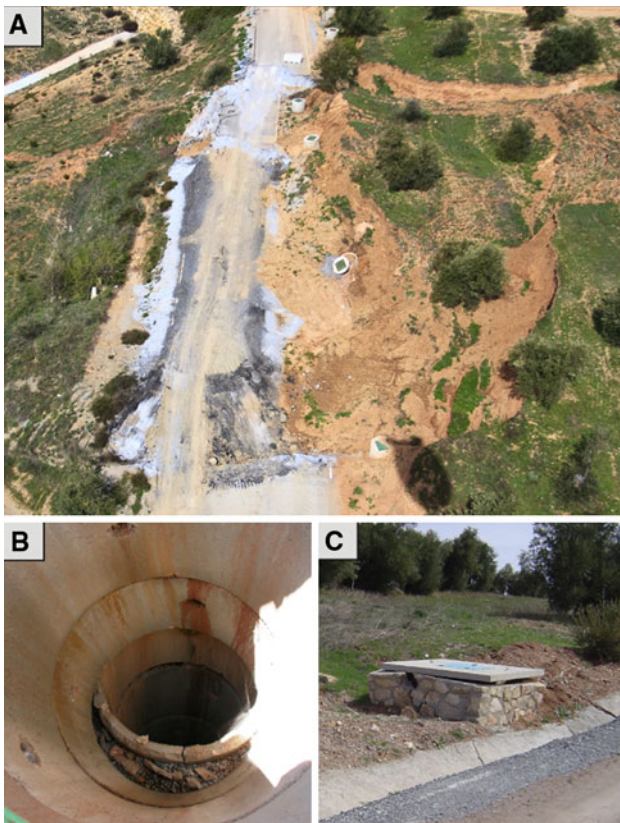
Fig. 8 a Aerial view of the first line of deep drainage wells and the old CN-342 road, which collapsed/moved during the 2010 landslide reactivation. b Broken well of the first line of drainage wells. c A damaged well in the second line of drainage wells
