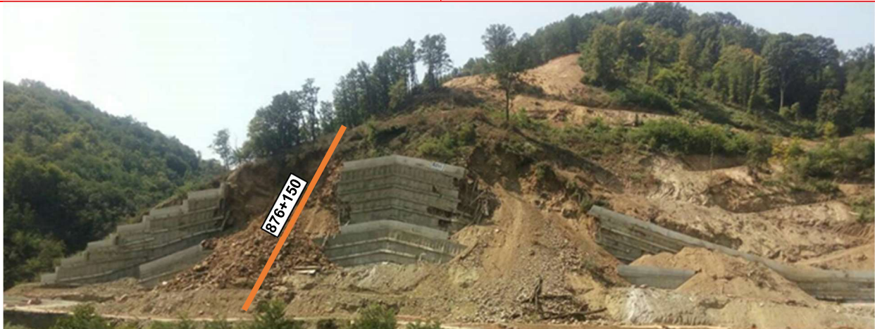
d) Failure of cut no. 2 in August 2018 (orange line indicates position of cross-section 876+150)
