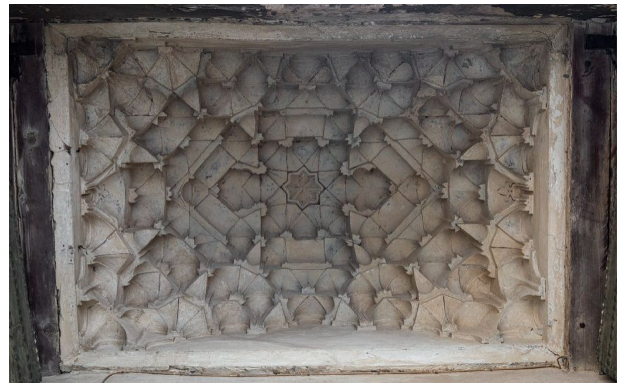
Lizard Gate Almohad vault, 12th century, Cathedral of Santa María de la Sede, Seville (Photo: Ramón Muñoz)
