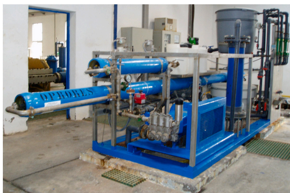
Fig. 1. SWRO desalination pilot plant.
