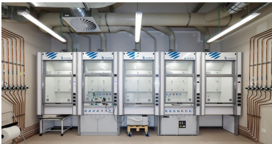
Figure 3.12. Frontal view of the fume hoods operating at the IR-35 facility.
