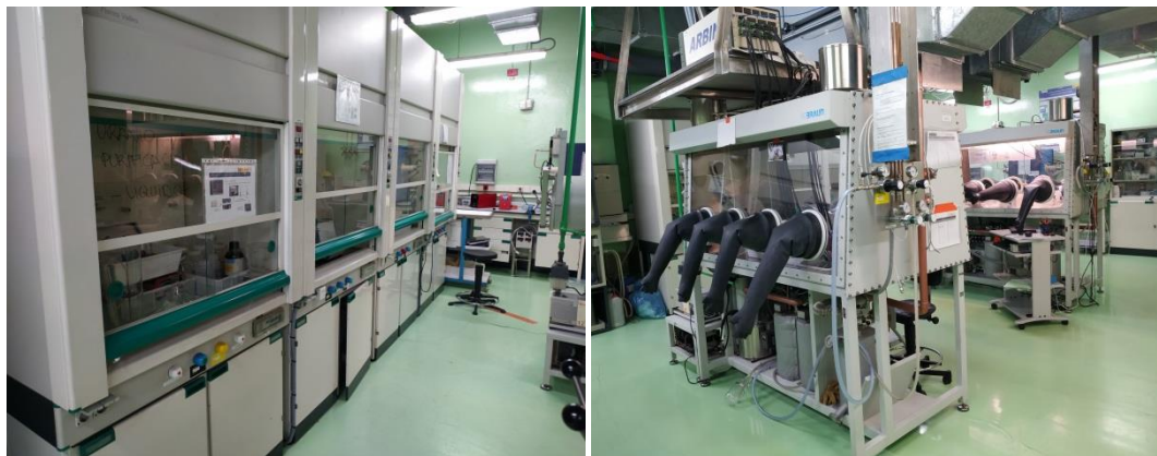
Figure 3.11. IR-30 Radioactive Facility, showing the fume hoods (left) and the glove boxes (right).
