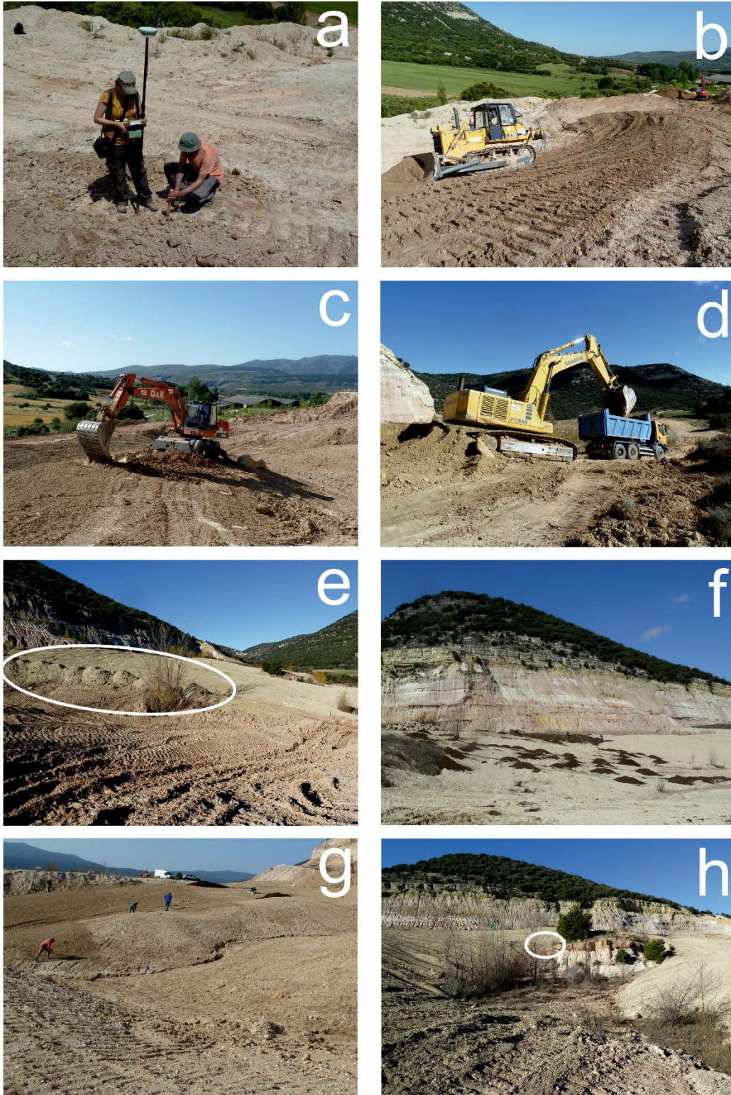
Figure 6. (a) Staking out the geomorphic design with DGPS; (b) D6 bulldozer regrading a scalloped hillslope; (c) excavator building a rock outcrop at the top of a ridge, to add geomorphic landscaping features; (d) excavator loading carbonatic colluvium to be used as subsoil; (e) mounds of carbonatic colluvium (white ellipse) being spread at the regraded surface; (f) mounds of organic matter (local sheep manure); (g) manual seeding and raking; (h) the white ellipse shows a local base level located at a stable sandstone ledge, visible at its right. This outcrop was also maintained, retaining geodiversity.
