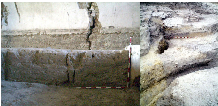
Fig. 20 Image inside the Ducal granary (XVIII century) (Fig. 2–4). It can be observed how granary walls and building foundations are affected by vertical cracks (left), in the landslide crown, with the contact between calcarenites rocks (yellowish color) and marls, along with anthropogenic sediments (grey color). This contact forms a preferential rupture surface that has affected the granary's flooring (right)
