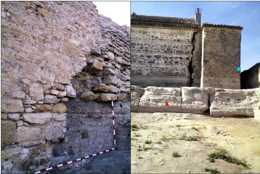
Fig. 21 Image from the Ducal granary (XVIII century). On the left, it is visible how the granary walls were adjusted to the remains of the previous fortress, compensating for earlier movements and surface irregularities and/or wall repairs. On the right, vertical cracks affecting the granary walls are visible
